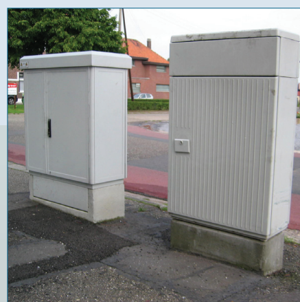
XDSL cabinet Next to copper cross connect
