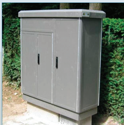
XDSL cabinet Overbuild copper cross connect
