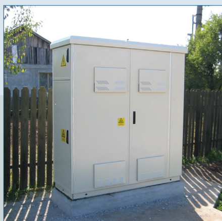
Remote central office
